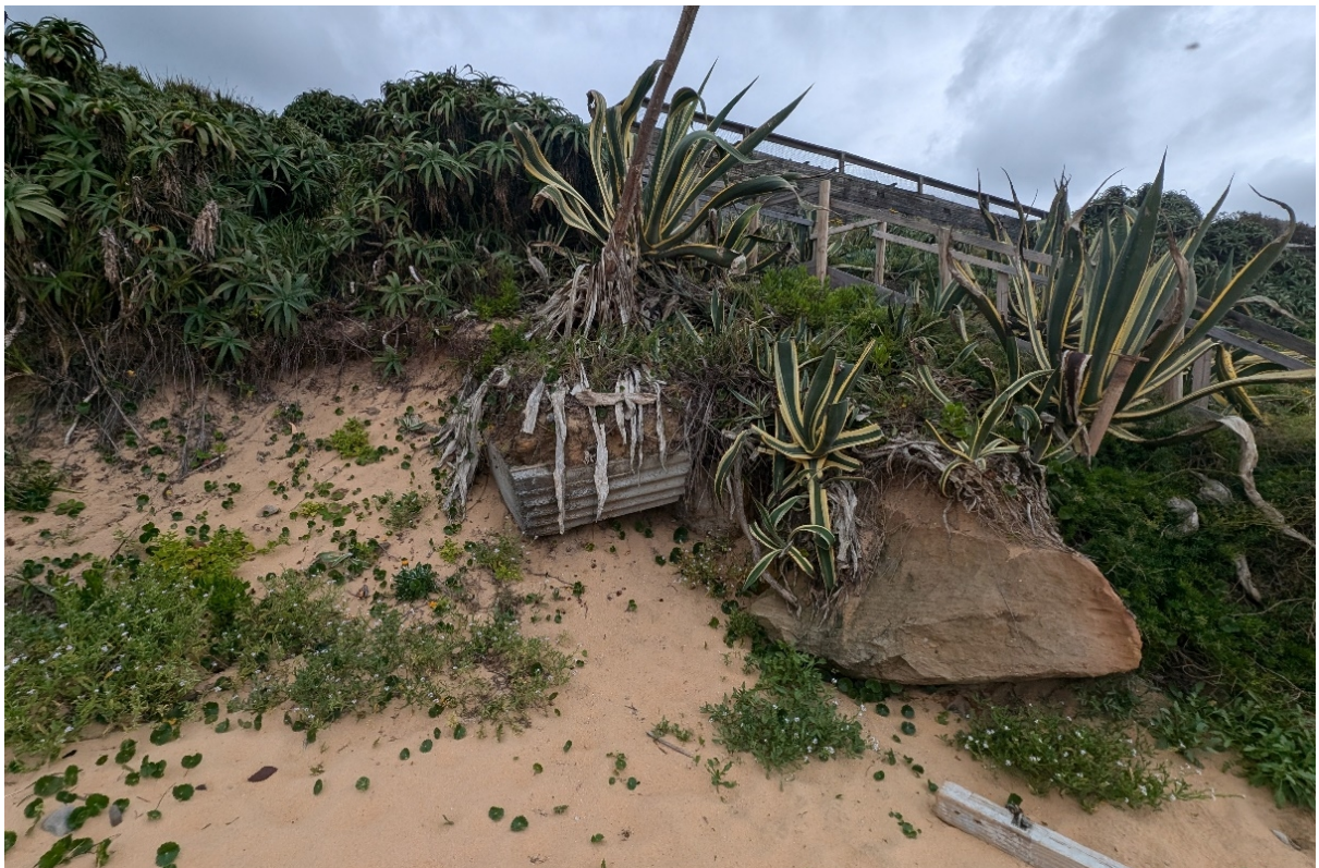
Figure 5 – Damage to rear of Calais Road properties
